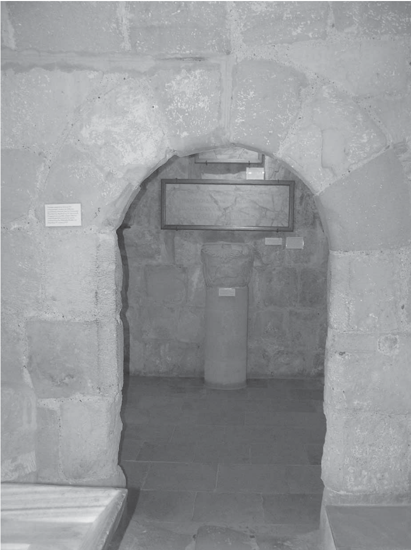
Fig. 32: Limassol Castle, upper level of cells, easternmost cell on north side, doorway showing signs of fire damage [M. Olympios].
